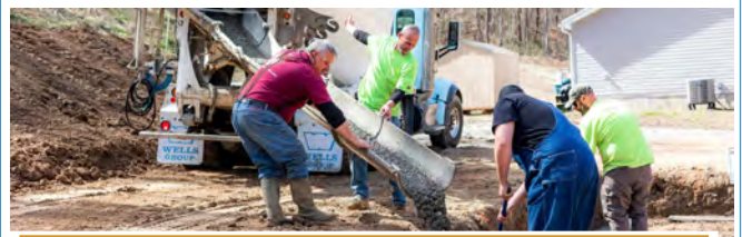
Concrete being poured for new homes funded in part by our Disaster Reconstruction Program.
